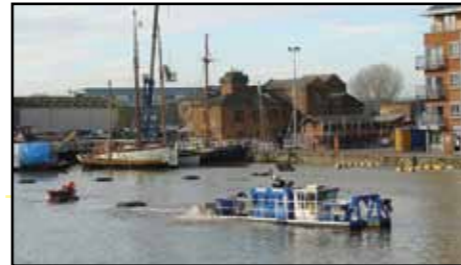
The Land and Water cutter suction dredger at work with a line of black floats supporting the discharge pipe leading to the small dry dock (picture courtesy of Hugh Conway-Jones).
